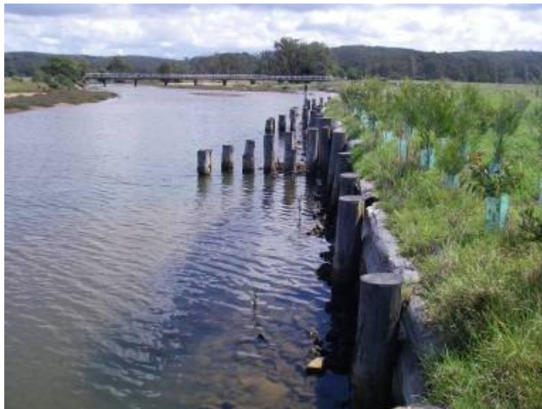
Figure 6a – Plants established on the banks above the log wall in March 2009. Also note the young mangrove plants growing through the rock beaching and the sea grass in the water (to the left of the rock beaching).
