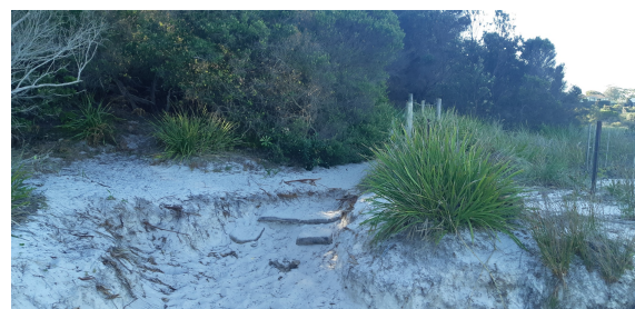
Figure 4: Example of erosion at accessway base
